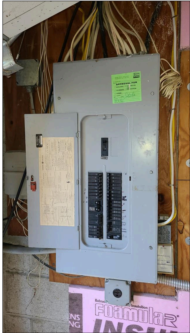
A. Item 2(Picture) Main panel
