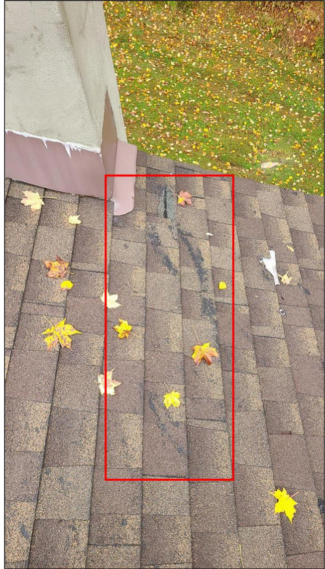
D. Item 6(Picture) Shingle damage
