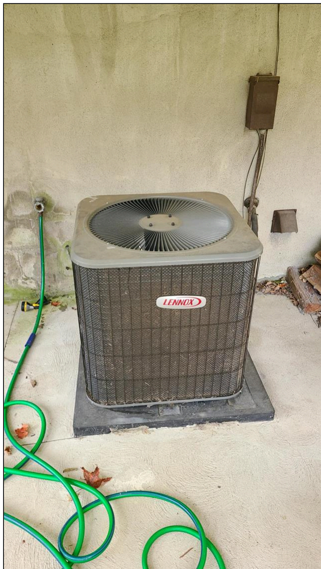
B. Item 1(Picture) A/C Condenser
