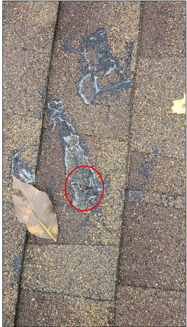
D. Item 4(Picture) Shingle damage down to the sheathing
