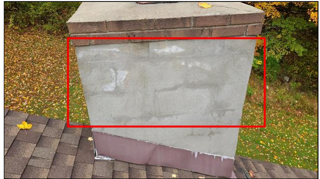
J. Item 2(Picture) Water intrusion
