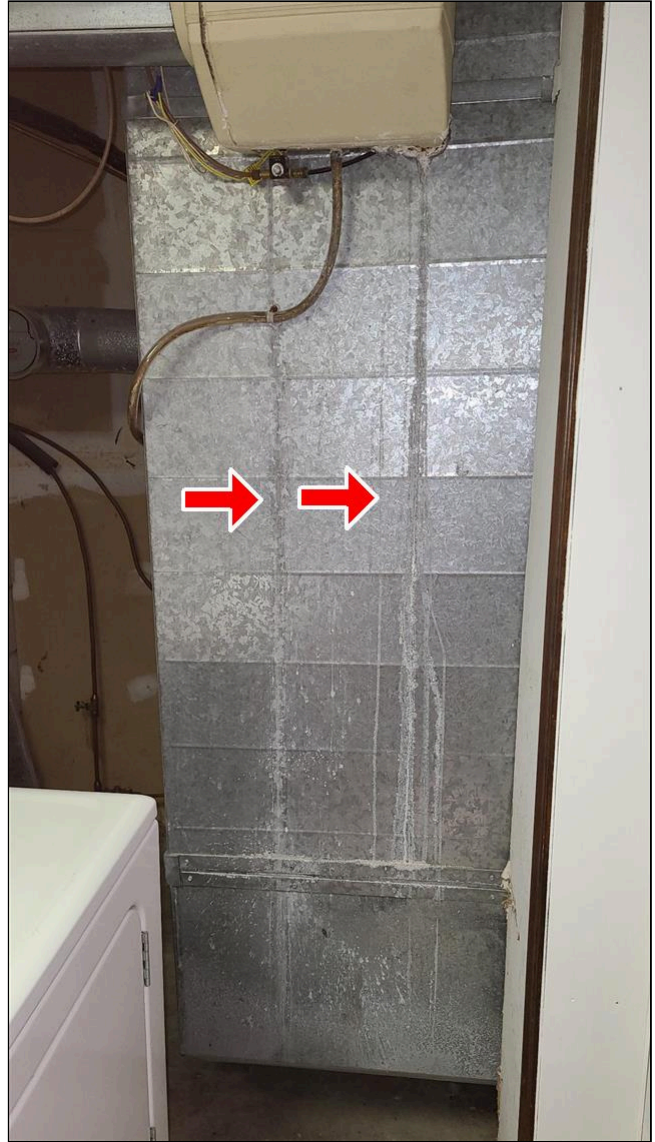
A. Item 4(Picture) Water marks
