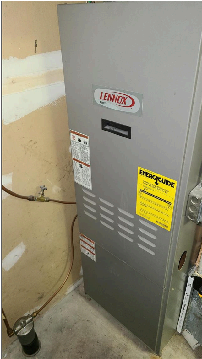
A. Item 1(Picture) Furnace
