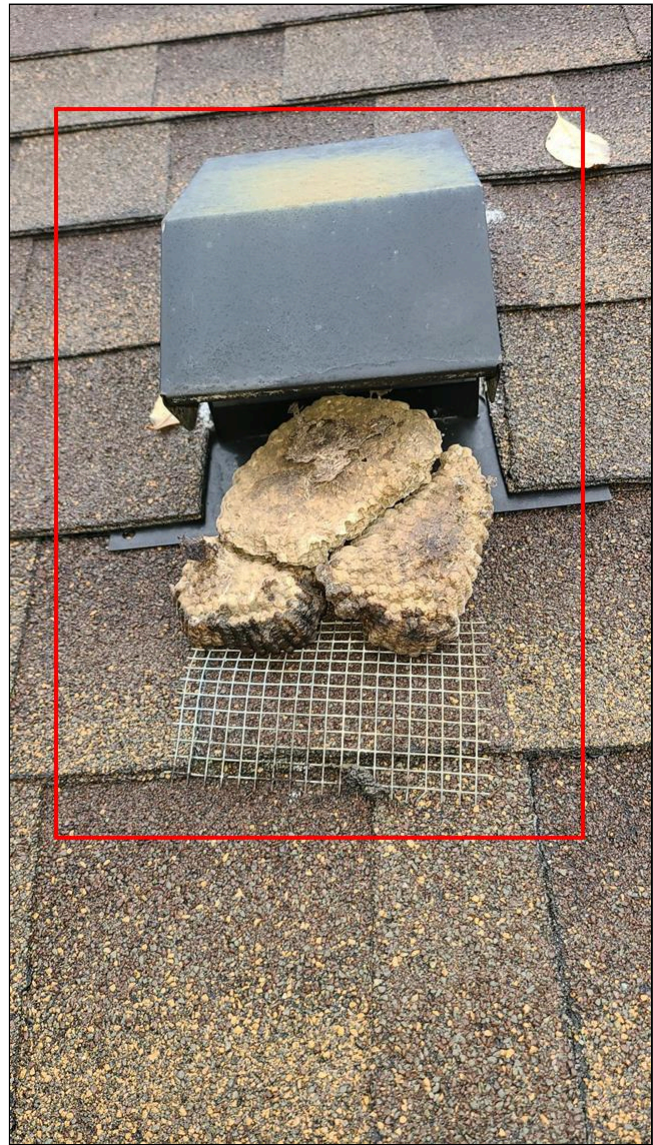
C. Item 2(Picture) Bath vent
