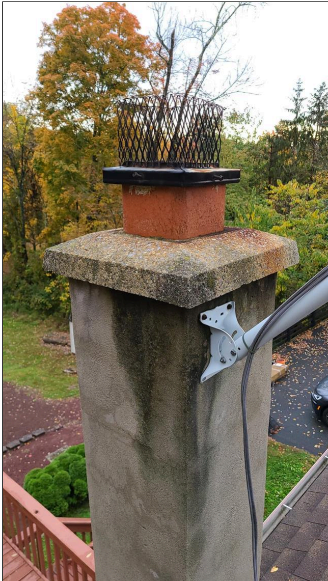
J. Item 3(Picture) Furnace Chimney
