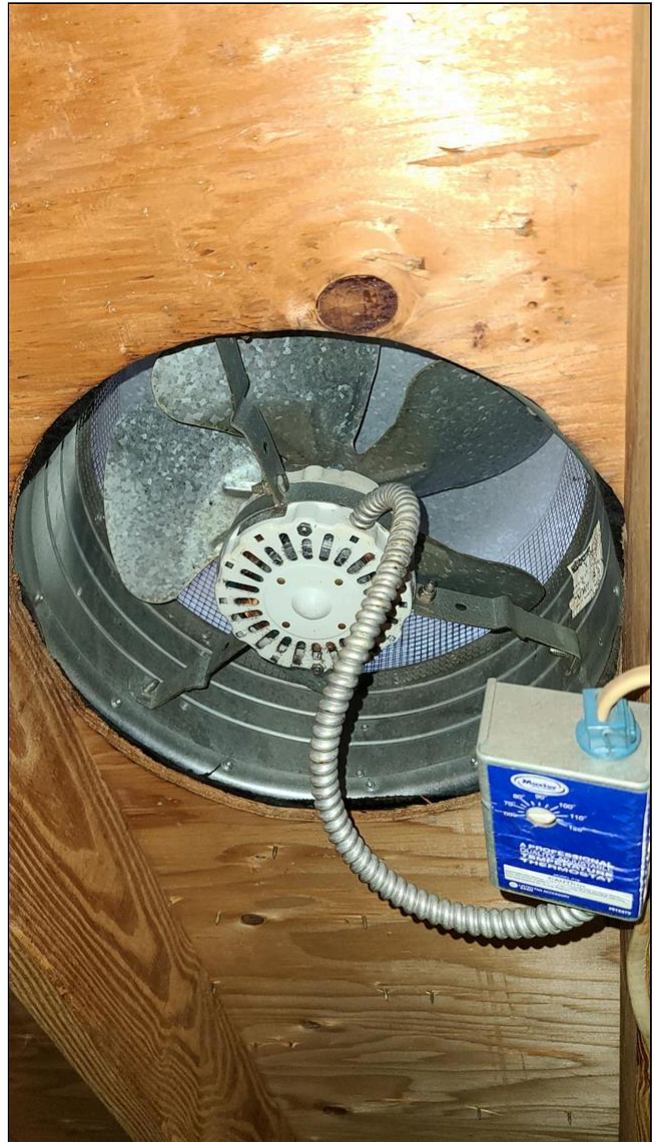
C. Item 8(Picture) Thermostatically controlled Attic roof vent most likely works as the blades turned freely.
