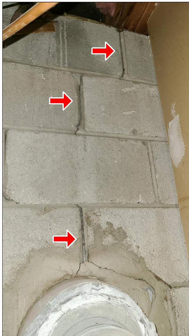
A. Item 2(Picture) Rear settling crack
