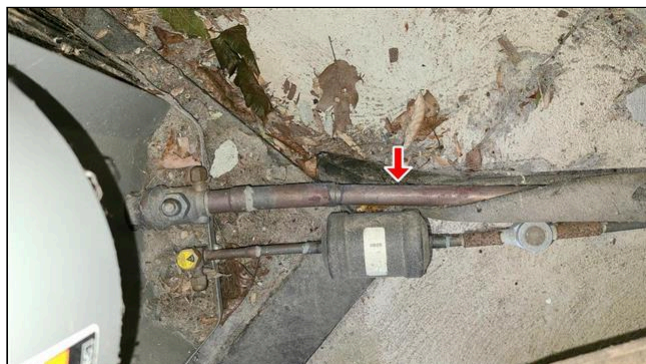
B. Item 2(Picture) Suction line
