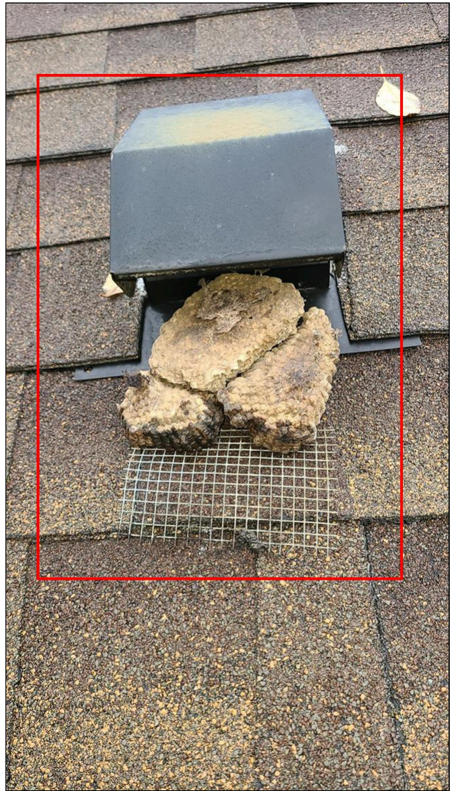
C. Item 2(Picture) Bath vent
