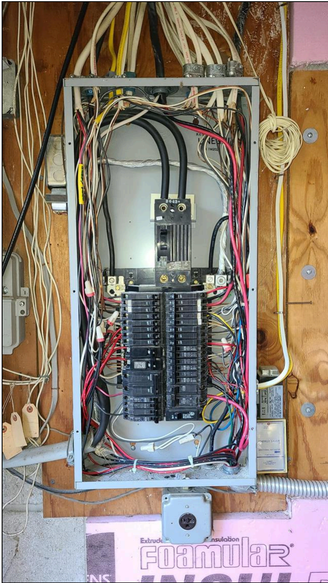
A. Item 3(Picture) Cover removed
