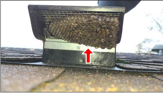
C. Item 3(Picture) Bath vent
