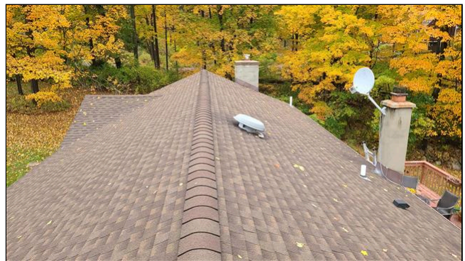
D. Item 8(Picture) Looking North
