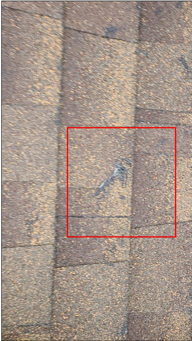
D. Item 3(Picture) Shingle damage
