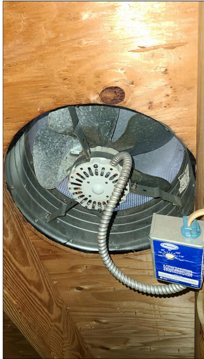
C. Item 8(Picture) Thermostatically controlled Attic roof vent most likely works as the blades turned freely.
