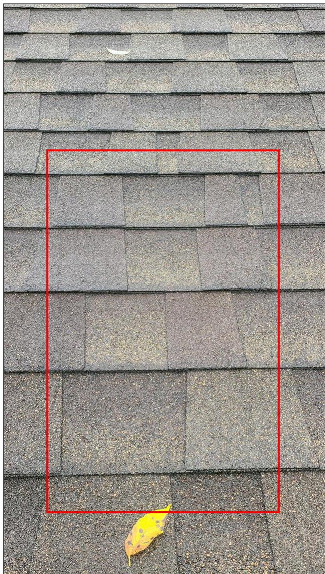
D. Item 1(Picture) The roof appeared to be in serviceable condition until I walked it. Looks to be about 12 to 15 years old, this type of shingle is warranted for 30 years.
