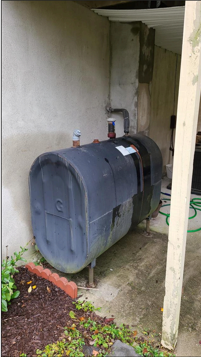
G. Item 1(Picture) 275 Gallon Fuel oil tank in the rear of the home.
