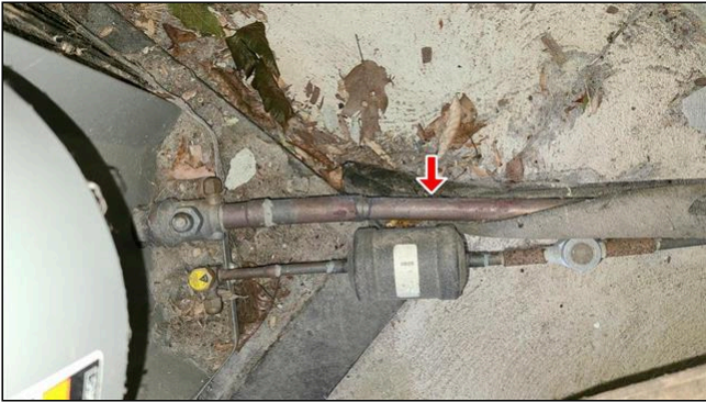
B. Item 2(Picture) Suction line
