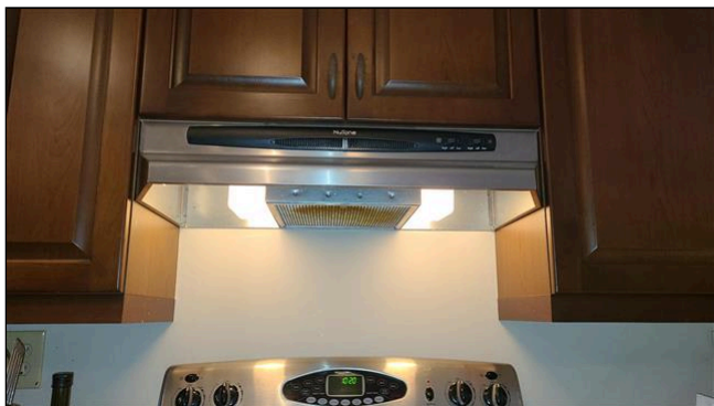
C. Item 1(Picture) Range hood
