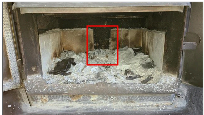
J. Item 10(Picture) Missing firebrick
