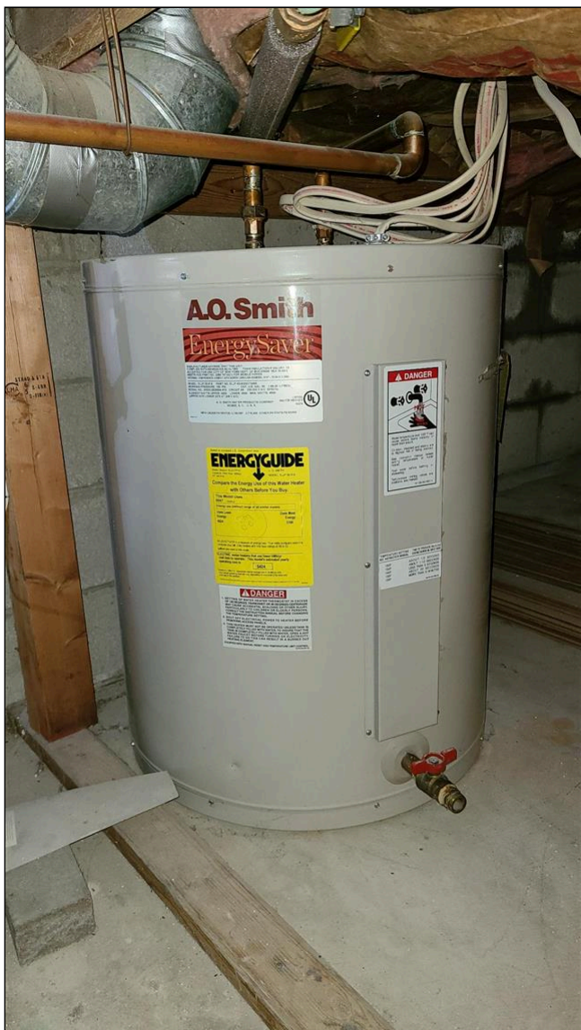
C. Item 1(Picture) Hot water heater
