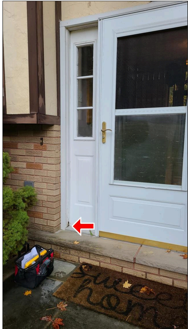
H. Item 2(Picture) Deterioration
