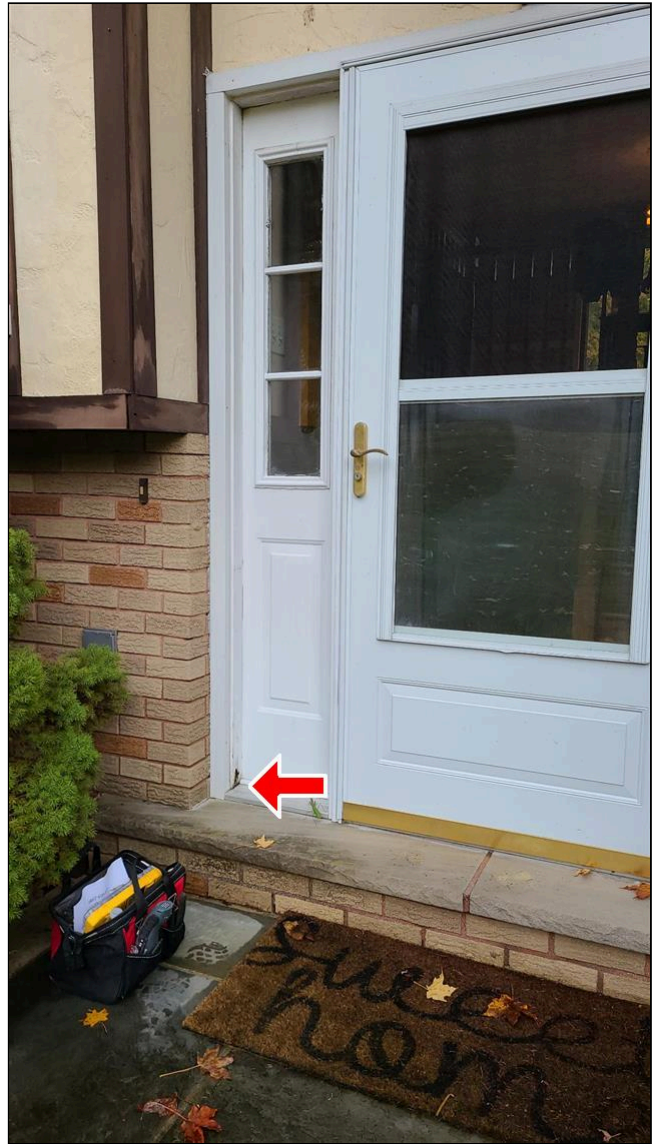
H. Item 2(Picture) Deterioration
