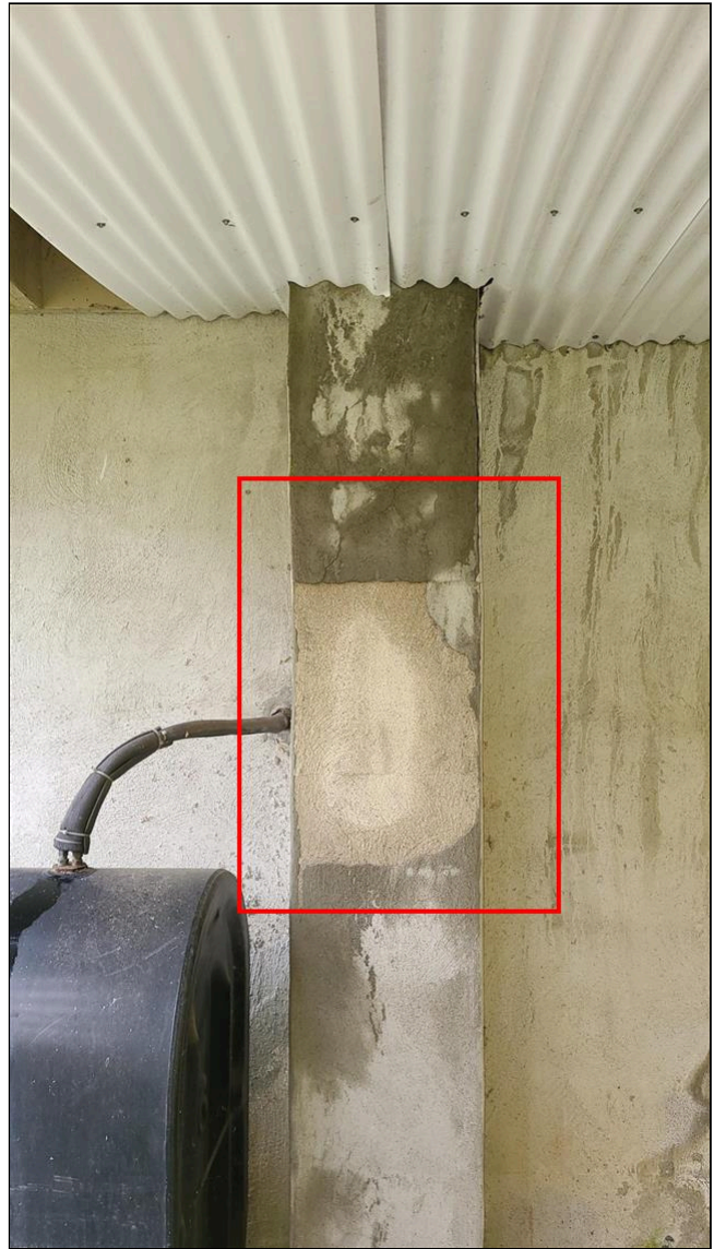
J. Item 8(Picture) Stucco damage
