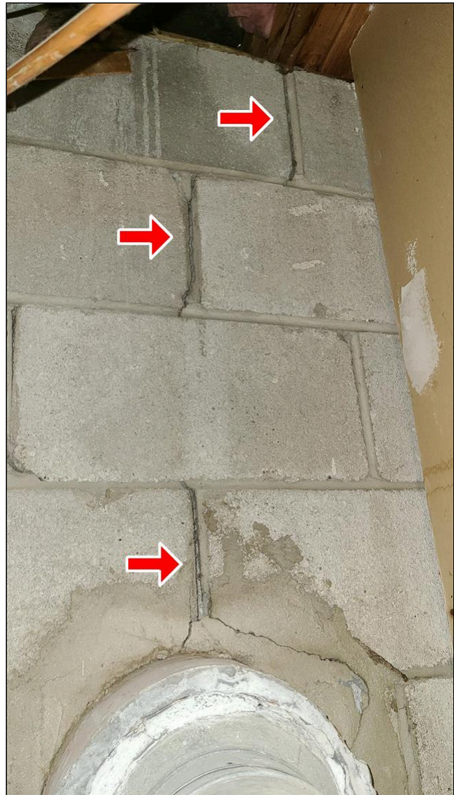
A. Item 2(Picture) Rear settling crack
