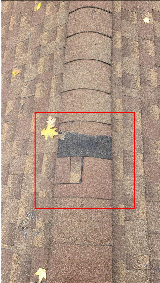
D. Item 5(Picture) Ridge damage
