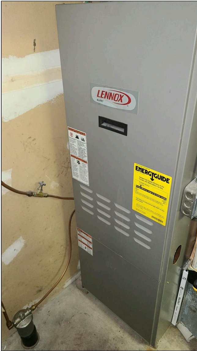
A. Item 1(Picture) Furnace
