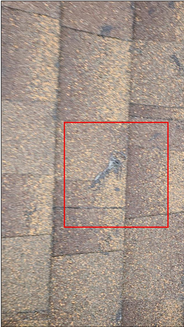
D. Item 3(Picture) Shingle damage
