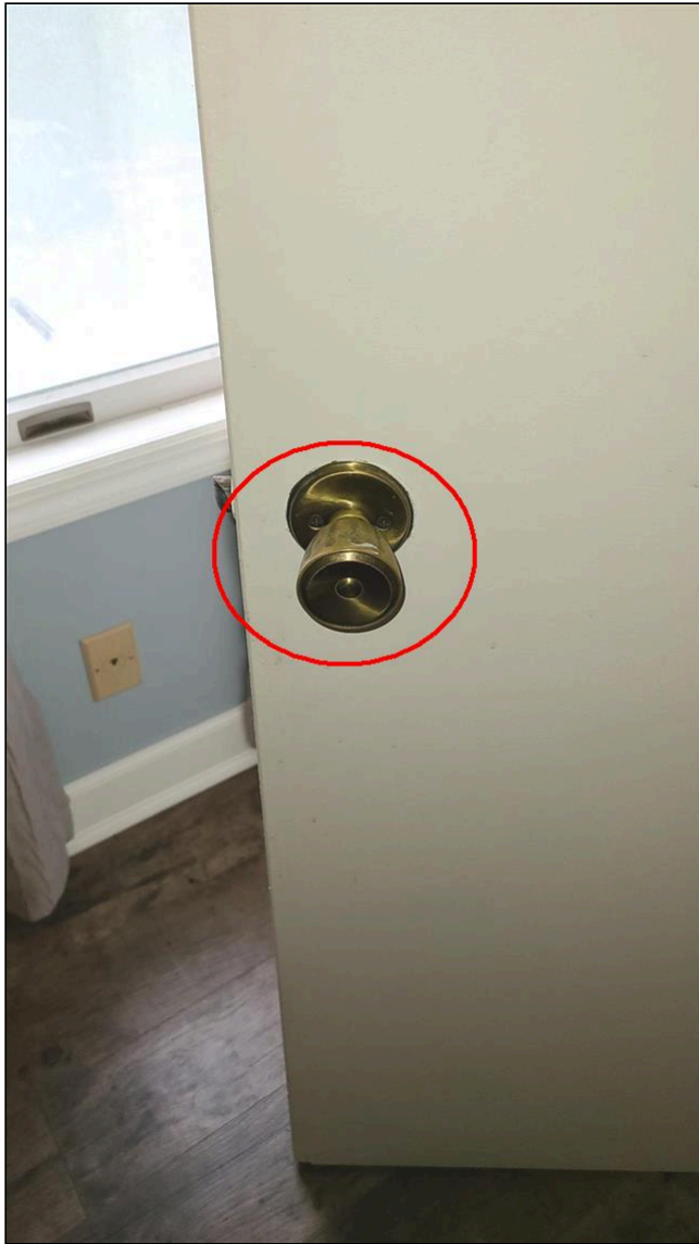
H. Item 3(Picture) The bathroom door handles do not lock.
