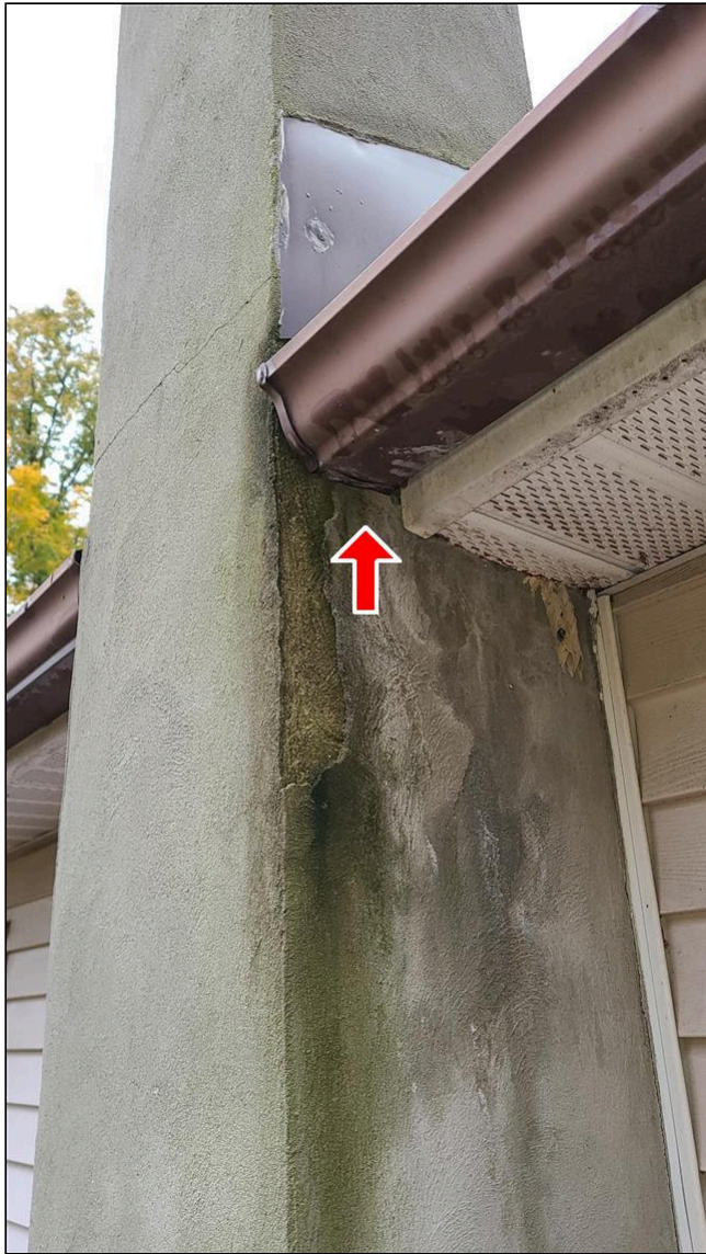
J. Item 5(Picture) Gutter leak damage
