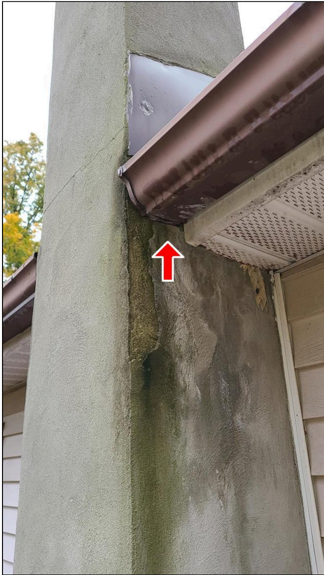
J. Item 5(Picture) Gutter leak damage
