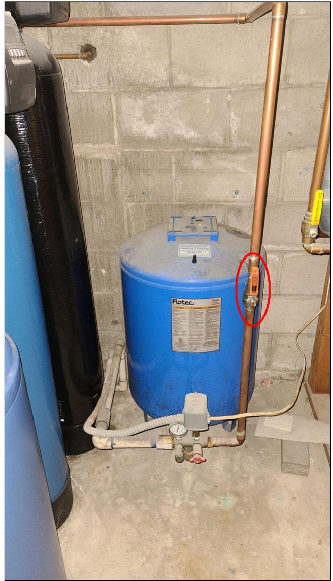
A. Item 4(Picture) Well pressure tank with main water shut-off circled.
