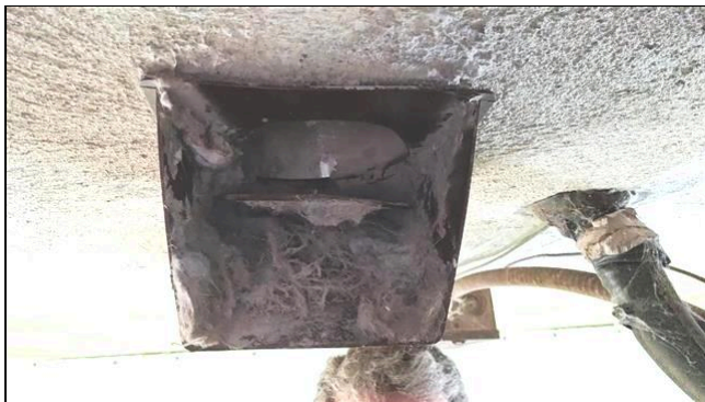
J. Item 1(Picture) Dryer vent needs to be cleaned
