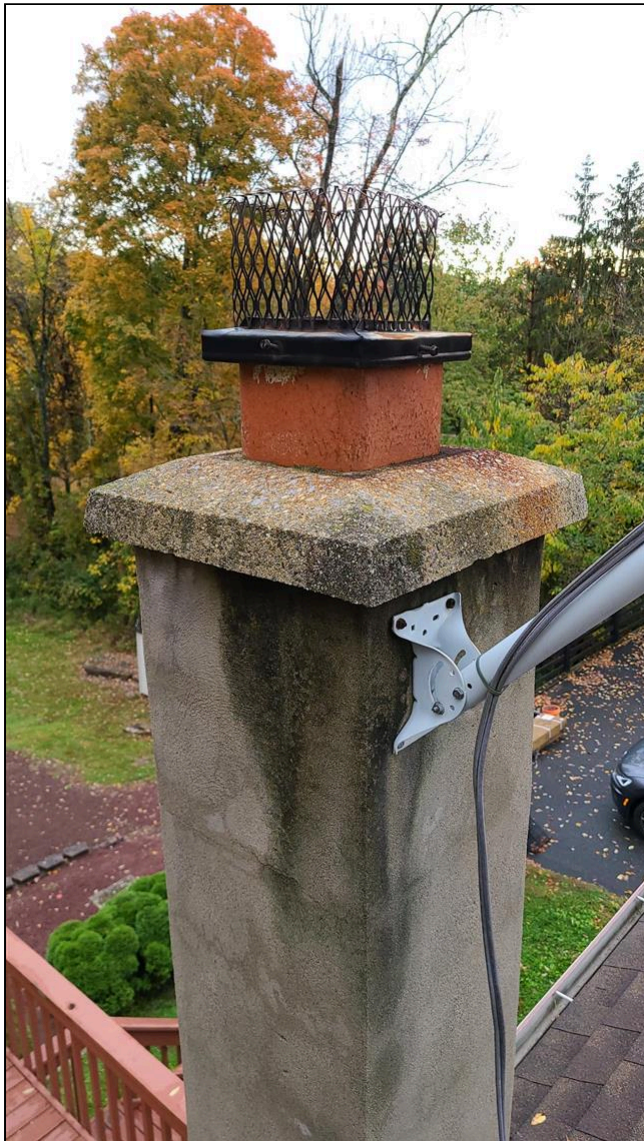
J. Item 3(Picture) Furnace Chimney
