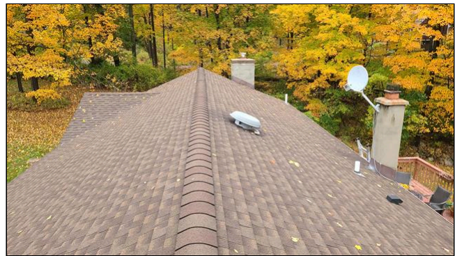
D. Item 8(Picture) Looking North
