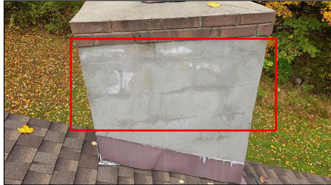
J. Item 2(Picture) Water intrusion
