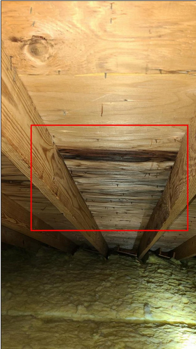
E. Item 1(Picture) Attic water damage
