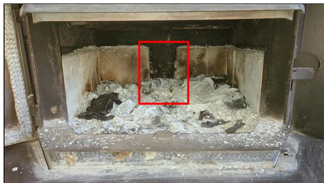
J. Item 10(Picture) Missing firebrick
