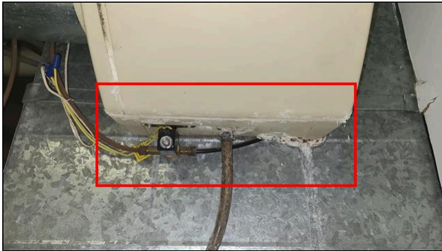
A. Item 3(Picture) Humidifier leak
