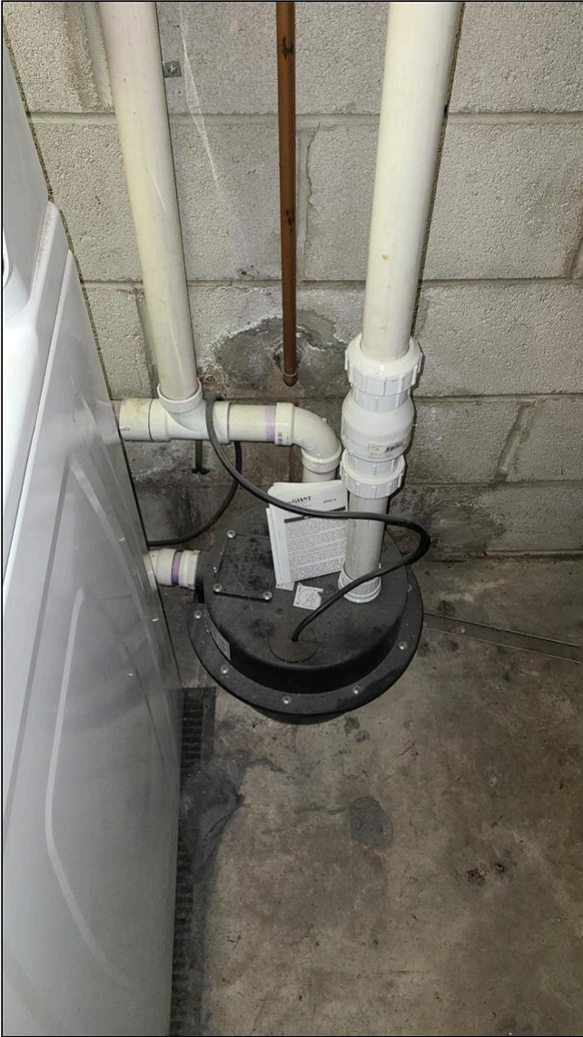
D. Item 1(Picture) Laundry Ejector pump
