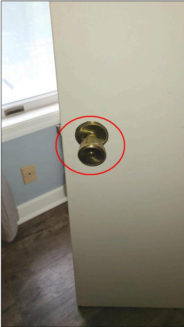
H. Item 3(Picture) The bathroom door handles do not lock.
