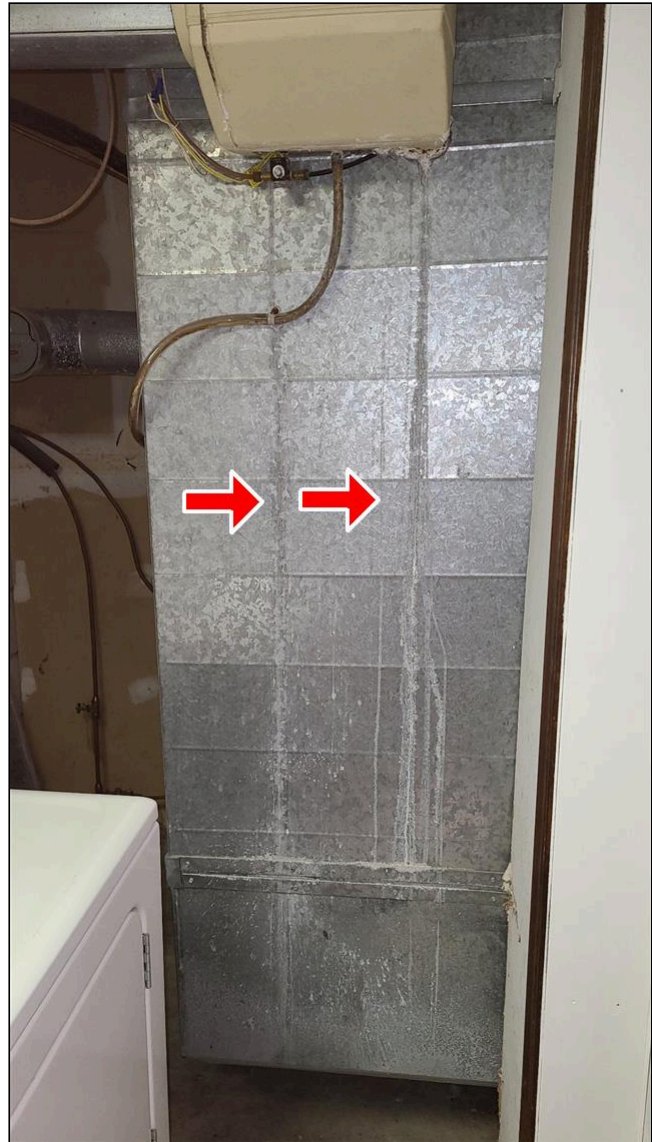
A. Item 4(Picture) Water marks
