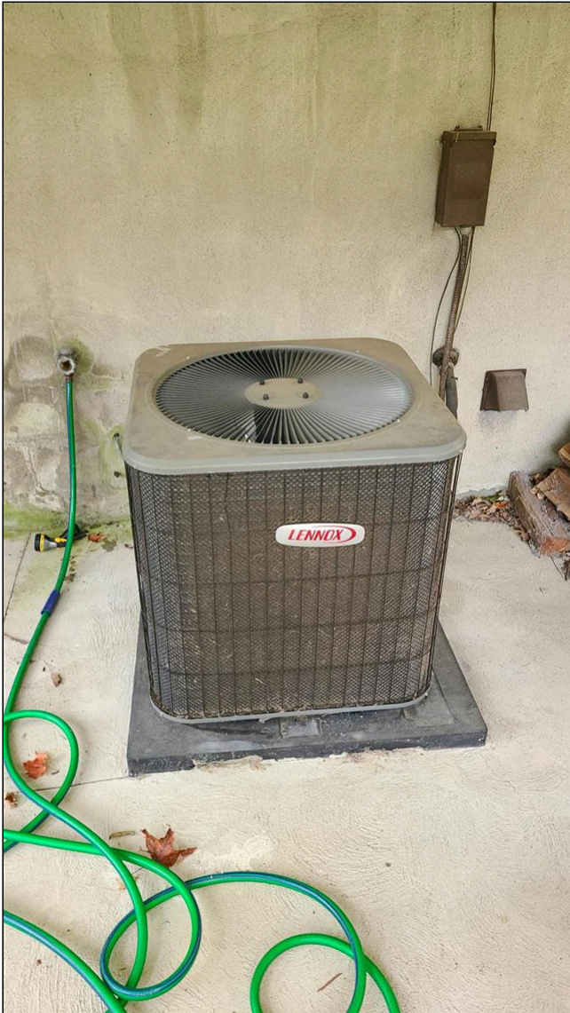
B. Item 1(Picture) A/C Condenser
