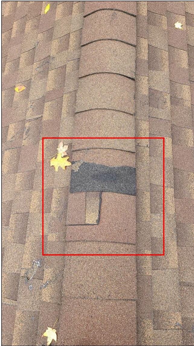
D. Item 5(Picture) Ridge damage
