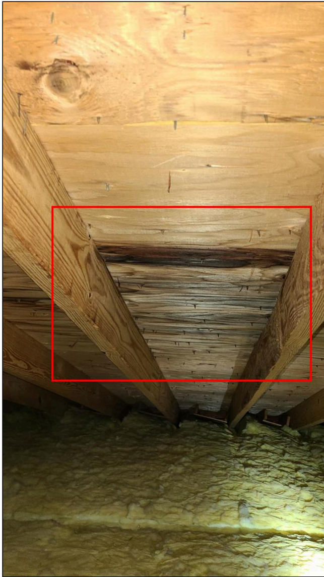
E. Item 1(Picture) Attic water damage
