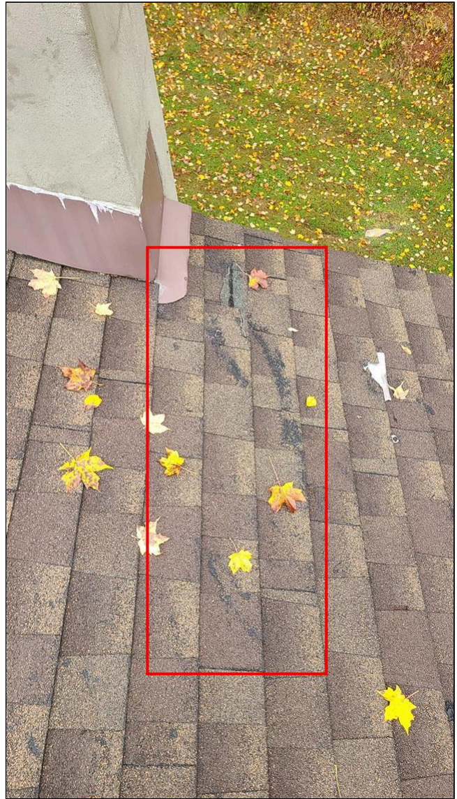
D. Item 6(Picture) Shingle damage
